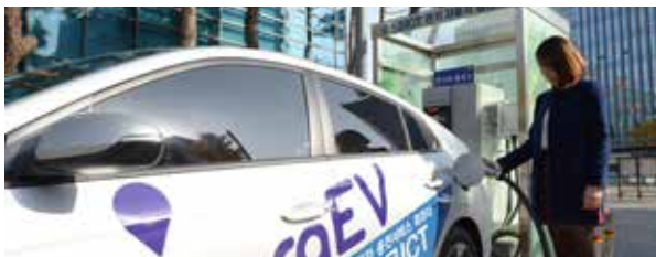
POSCO ICT's EV Charging Station
