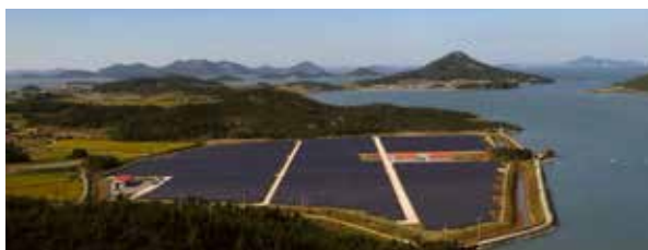
POSCO Energy's Sinan Solar Power Generation Complex(third phase)
