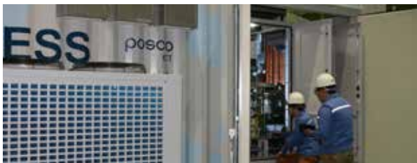
POSCO ICT's Pohang ESS Test Center(144MW)
