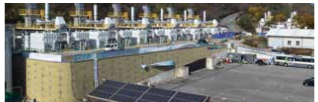
POSCO Energy's Noeul Green Energy Factory in Seoul
