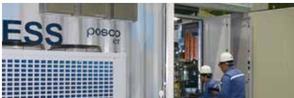
POSCO ICT's Pohang ESS Test Center (144MW)
